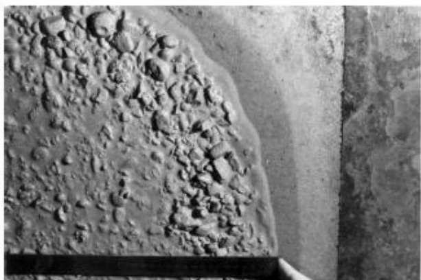
(b) Lack of cohesion in the concrete has resulted in grout segregation round the perimeter of the sample
